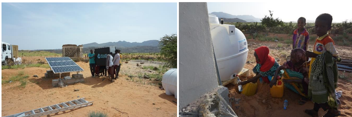
Installing a REvIVED water desalination unit at the village of Beyo Gulan, Somaliland (photo credits: Phaesun).
